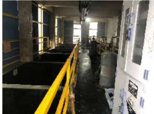
(f) 废液暂存区围堰
