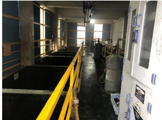
(f) 废液暂存区围堰
